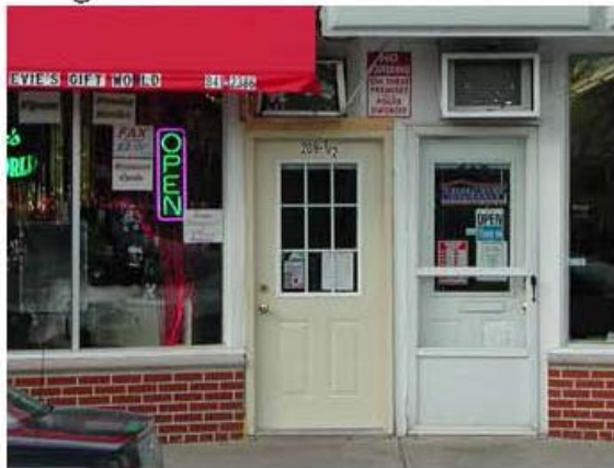
Prohibited: Residential Grade Doors on Commercial Buildings.
